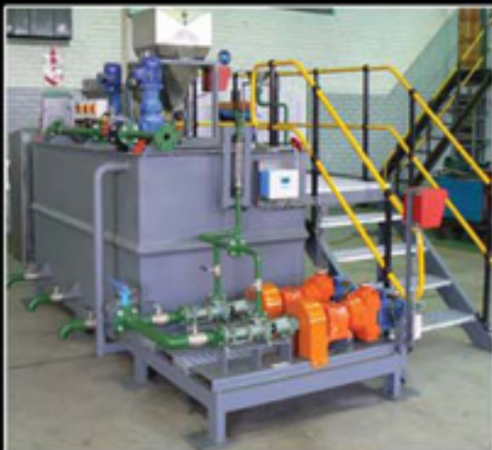
MIP-200 Flocculant Plant
