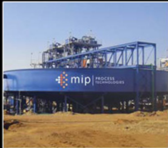
26m \phi Thickener in operation
