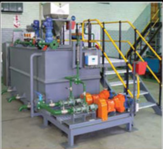
MIP-200 Flocculant Plant
